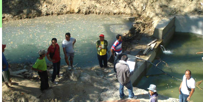
Irrigation project in Tayum, Abra under the Irrigation Support Project for small tobacco farmers. NTA Abra
