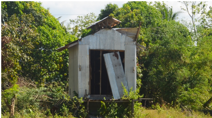
A multi-purpose curing barn damaged by Lawin in Bucay, Abra.
