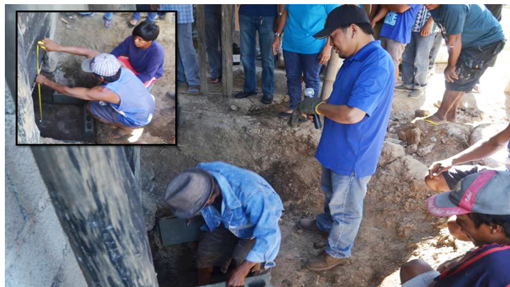
Engr. Abella (standing in blue shirt) observes the construction of anawang furnace at a flue-curing barn in Piddig, Ilocos Norte
